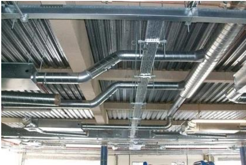
HVAC DUCTING SYSTEM
