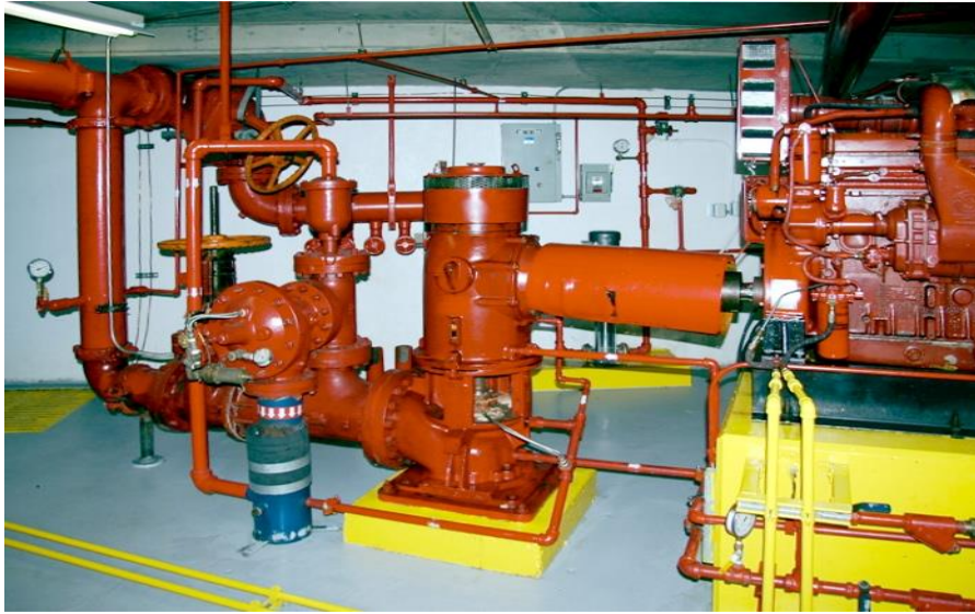
FIRE PUMP – JOCKEY & MAIN FIRE PUMP AND ACCESSORIES.
